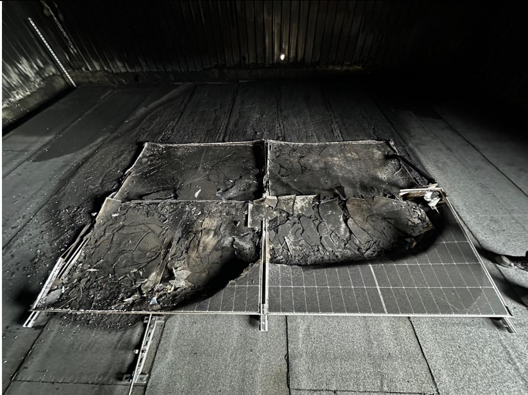
Figure 26: Damage of PV panels after test with PIR insulation roof.
