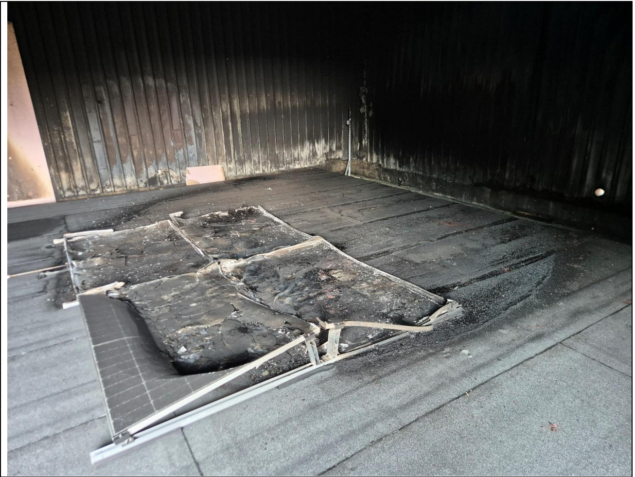
Figure 47: Damage of PV panels and roofing membrane after test with Stone wool insulation Roof.
