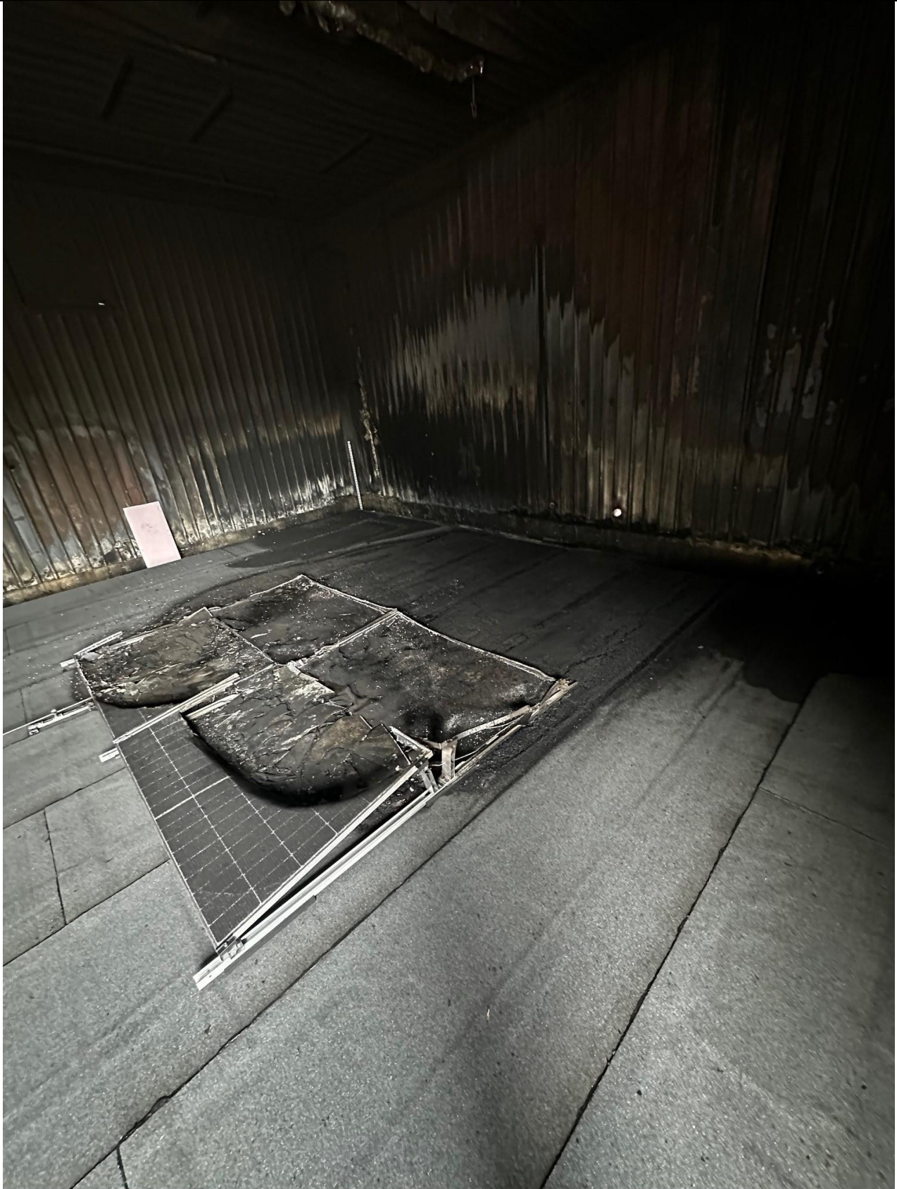
Figure 25: Damage of PV panels and roofing membrane after test with PIR insulated roof.
