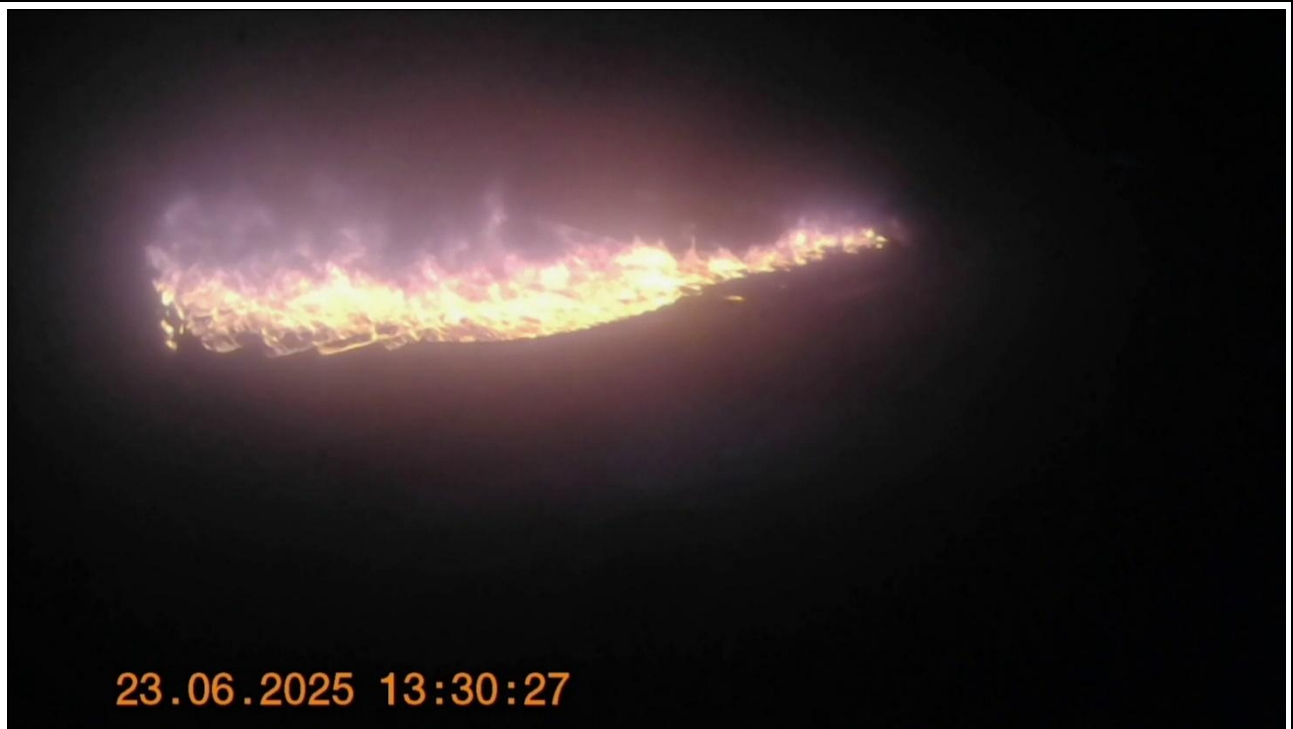
Figure 22: Fire exhibits further spread across roof assembly (Camera 2)
