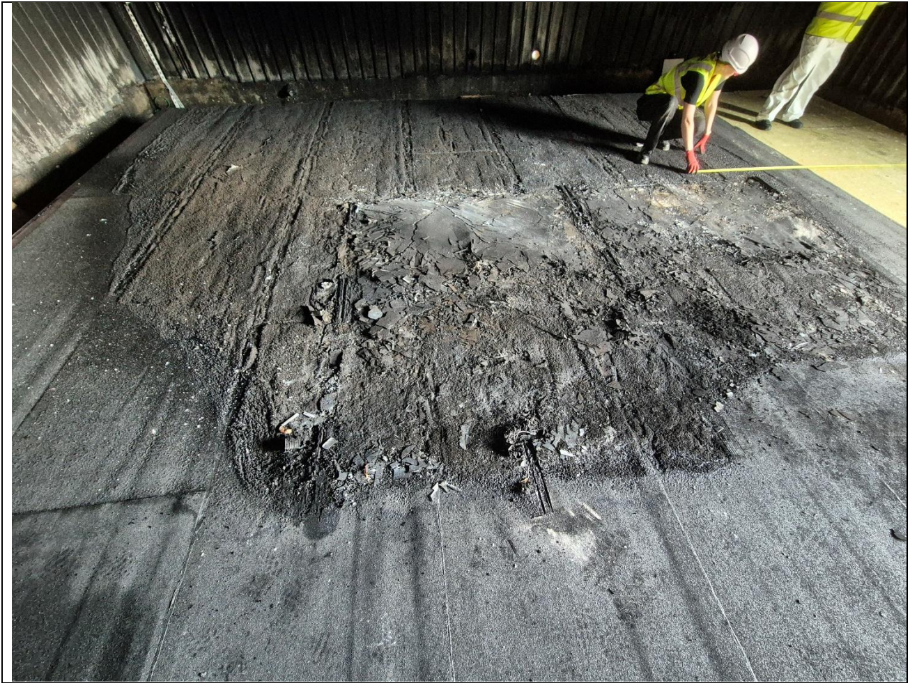
Figure 48: Damage of roofing membrane after test with Stone wool insulation roof.
