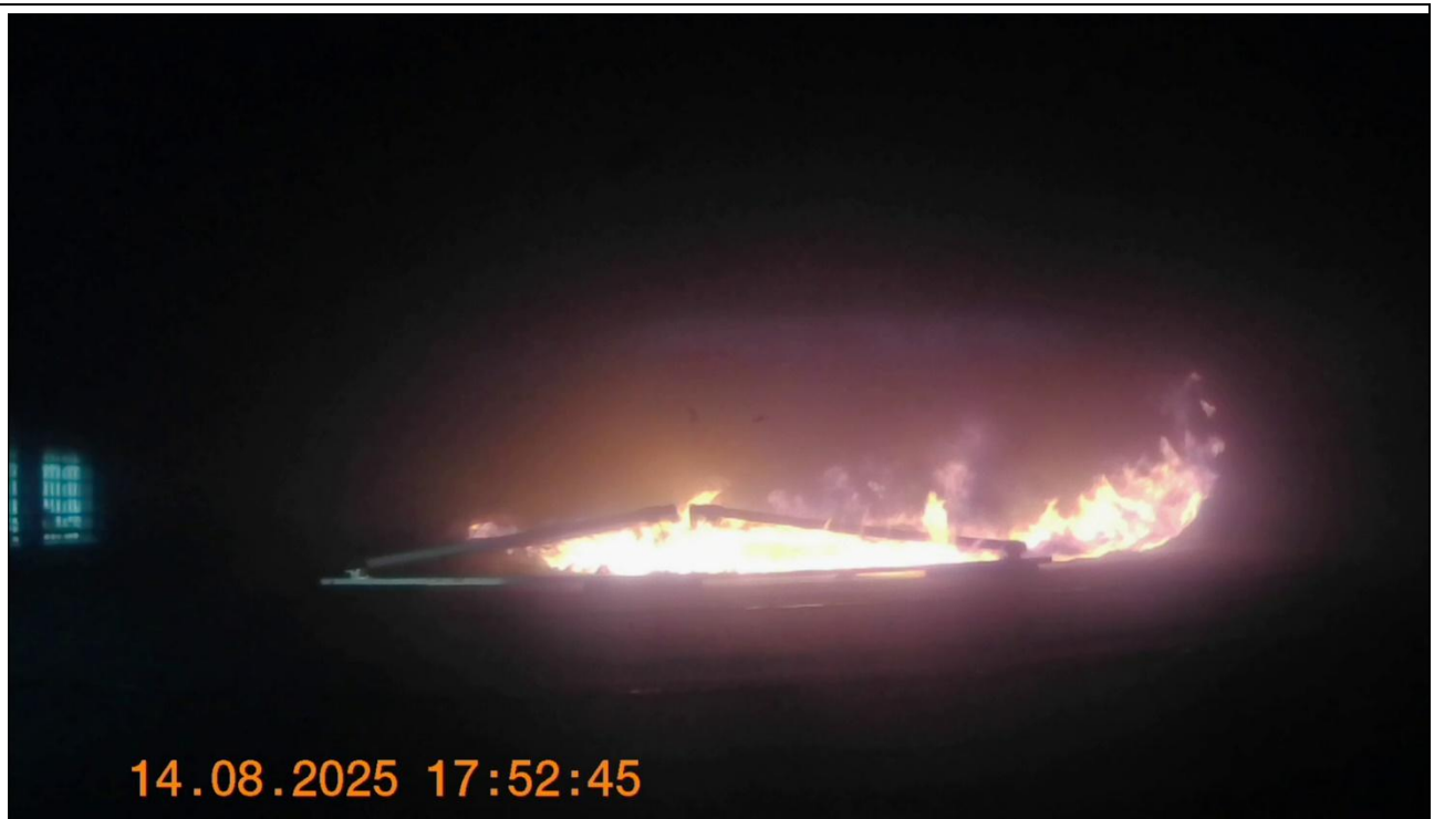
Figure 43: Fire continues to spread across roof assembly (Camera 3)
