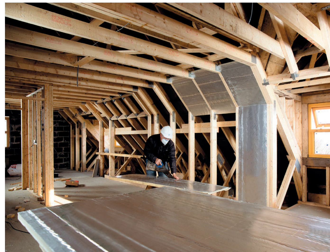
Above: Roof installation of PIR Boards; Left: Flat roof boards being installed: “To achieve more thermally-efficient building envelopes we must have a fabric-first approach.”
